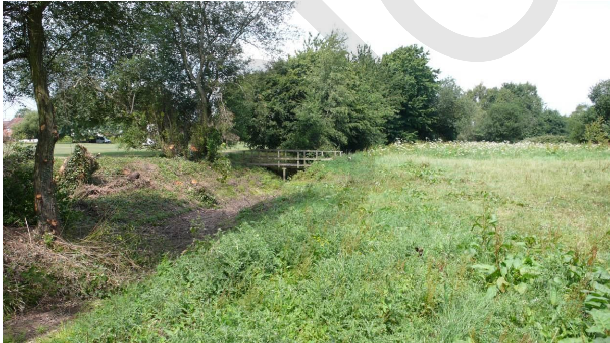
View north looking along the drain line (12). Recently thinned and opened up locally.
